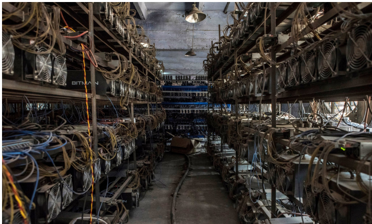
Figure 14: Racks of machines mining Bitcoins and Ether at a server farm in Guizhou, China, June 2017. Current hash rate estimated at 10 million trillion SHA256 hashes per second! Over USD1.1 billion of electricity consumed annually, about the use of Ecuador. Sources: photo Gilles Sabrié for The New York Times, https://blockchain.info/charts/hash-rate , https://digiconomist.net/bitcoin-energy-consumption
